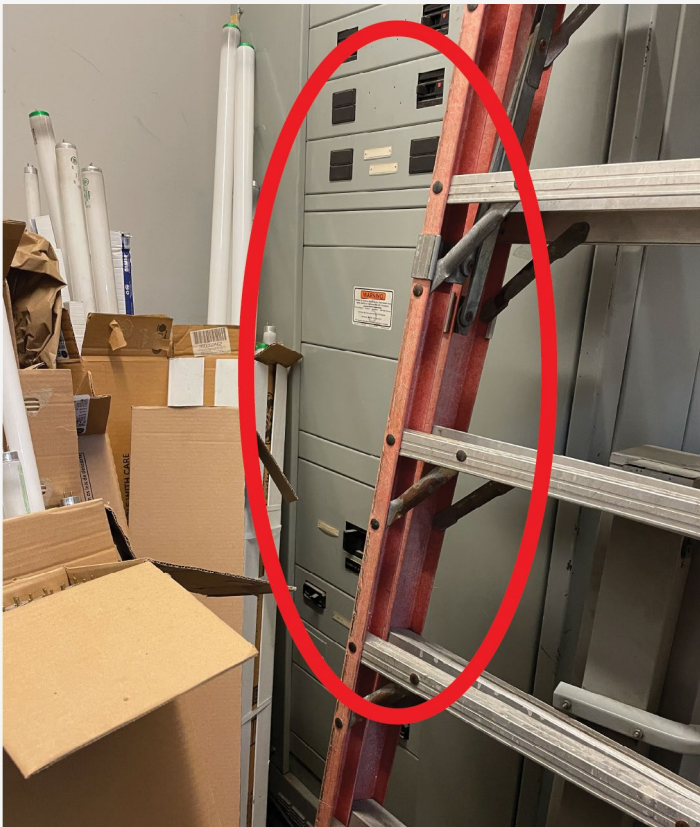
Figure 2. Blocked Electrical Panel
